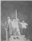
NEW AIR-OPERATED valve actuator at largest tank No. 914. VALVE NOBO opera cu aire na tanki mas grandi No. 914.
